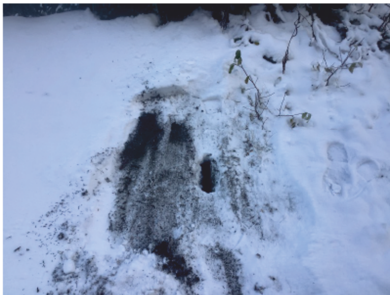
Right bank panel 1 ballast wall and panel damage
